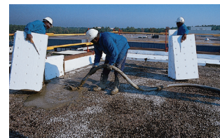
Decreasing thicknesses of Insulperm Insulation Board form the slope-to-drain contour of the finished system.
