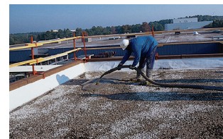
On this reroofing project, a thin slurry coat of lightweight insulating concrete is poured in place, correcting substrate irregularities and bonding the Insulperm Insulation Board to the substrate.
