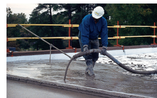
A top layer of insulating concrete is placed over the Insulperm, filling the holes in the Insulperm and locking it into the system without the use of fasteners.
