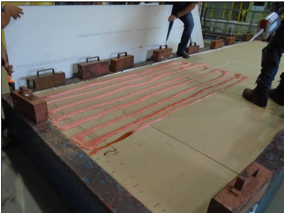
Photo C-6 – DensDeck® Prime cover board ribbon adhered with Parafast Insulation Adhesive C and weights applied on top
