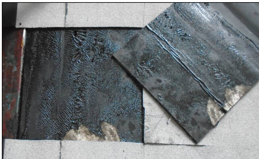
Figure 5 – Adhesive failure between the base sheet and insulation board
